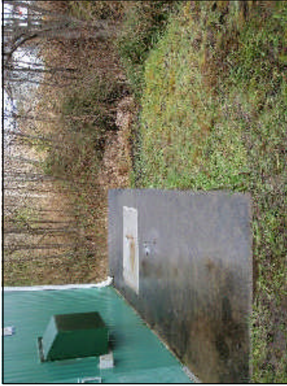
Photo 1. Location of the spill at the Peel Street and Beaver Harbour lift station.
