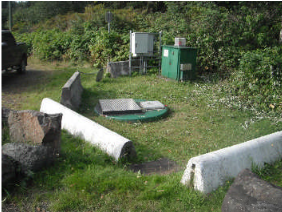
Photo 1. Pioneer lift station observed on August 25, 2011 following the events of the grey water spill into the nearby Quatse River.
