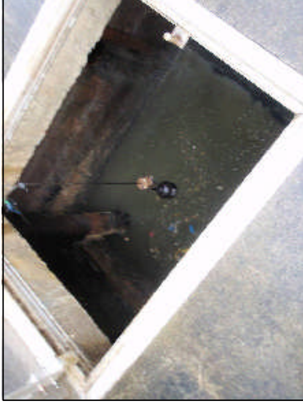
Photo 2. The overflow of the wet well (on this photo) was at the origin of the spill.
