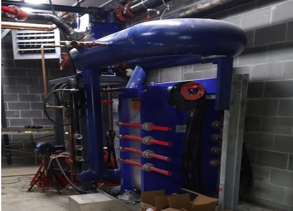
New Plate and Frame Chiller
