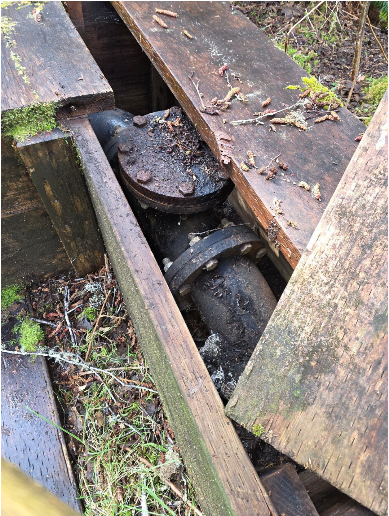
Attachment 5 Water Pipe.
